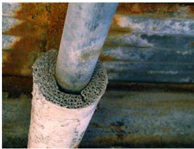
Asbestos pipe insulation
